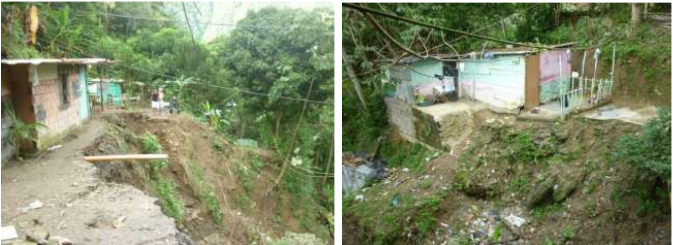
Vargas state, near Pastor's Fuentes church in Caraballeda - Houses at risk, part of them already felt down.
